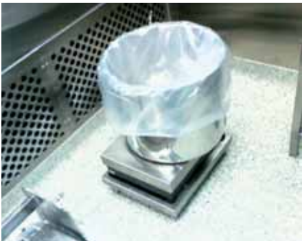
Photo taken on site after installation and commissioning of the system
